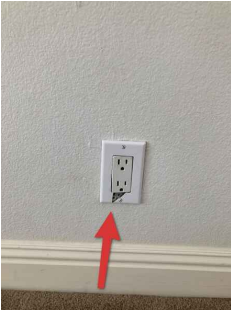
Broken cover plate
