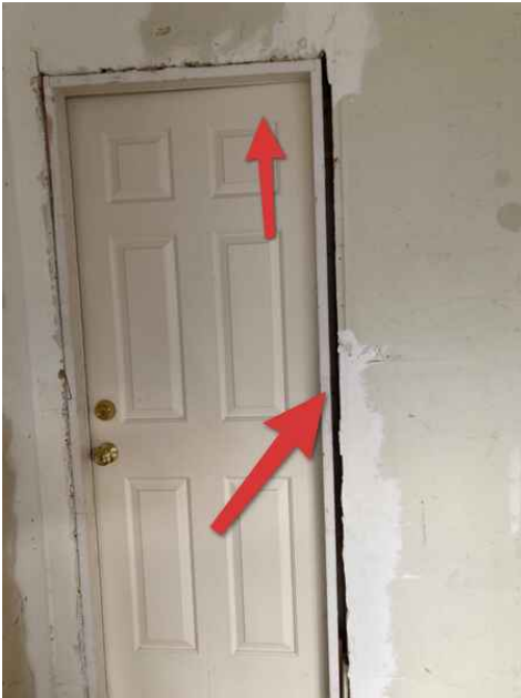
Open gap, no automatic closing mechanism
