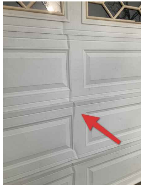
Damaged garage door
