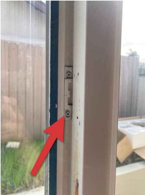
Window missing lock mechanism
