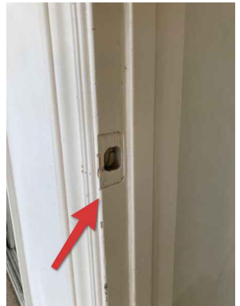
Strike plate missing
