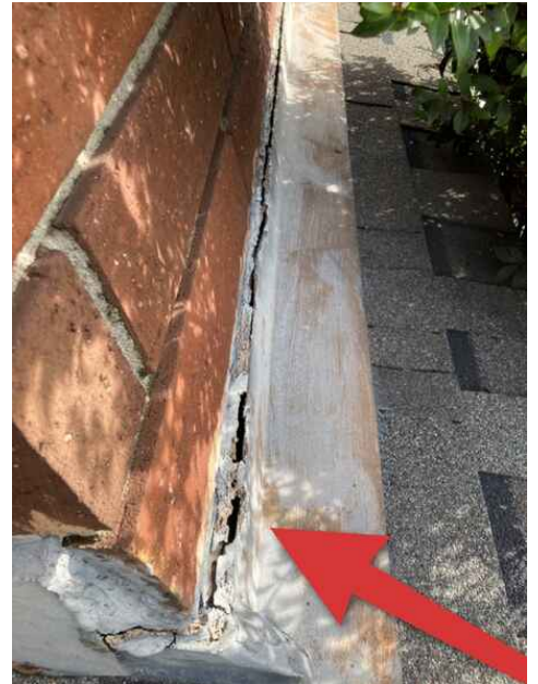
Flashing separating from chimney
