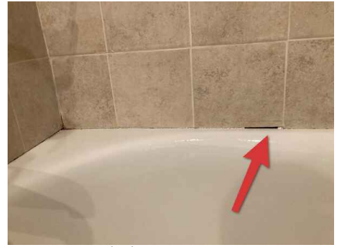
Gaps around tile
